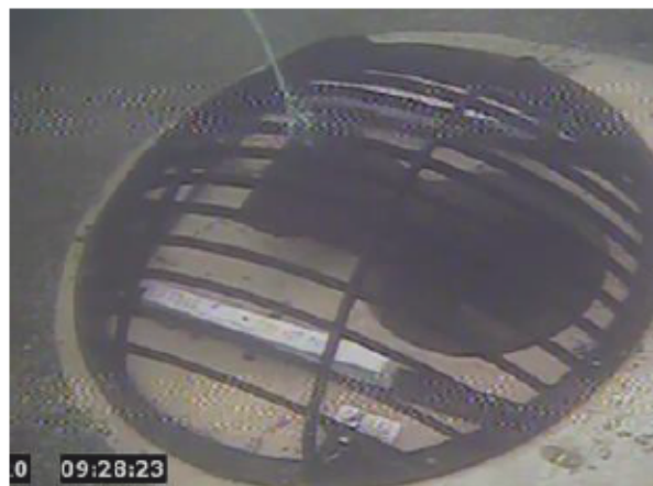
Figure 11-1 Installed Diffuser Port with Guard
