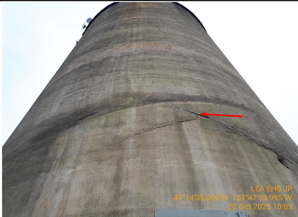
Figure 2. Asbestos-Containing Black Mastic on Exterior Concrete Wall of Silo.
