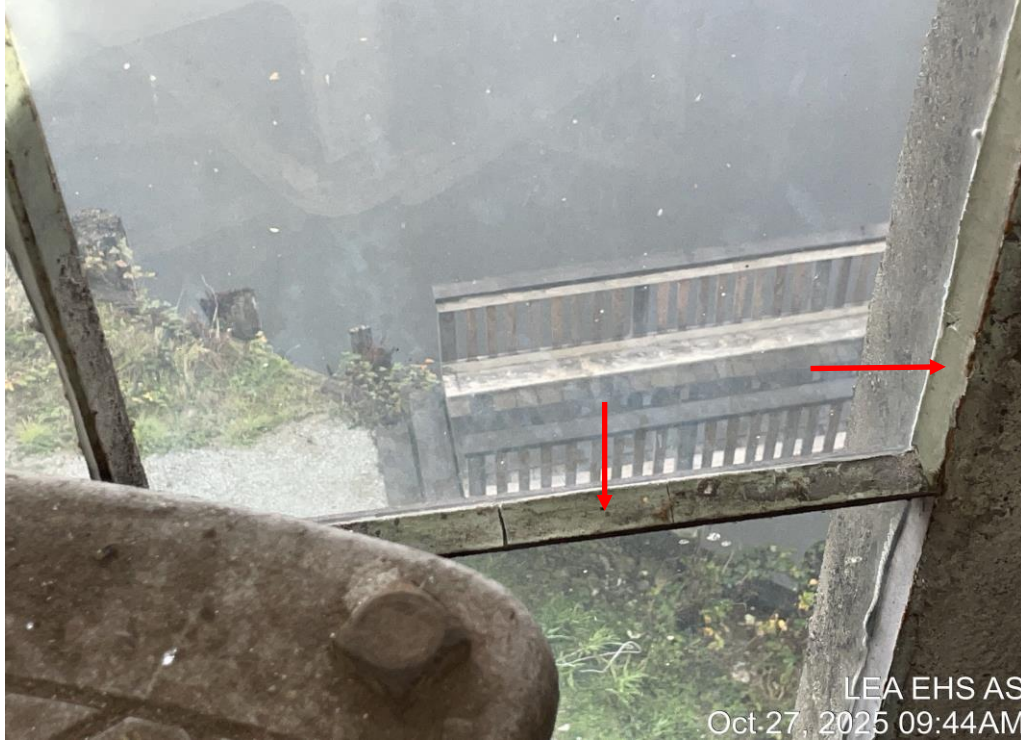
Figure 1. Asbestos-Containing Off-White Window Putty - Interior.
