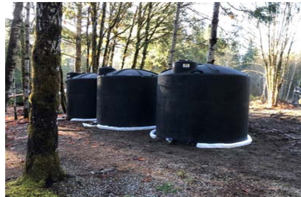
Photo 11. Containment holding tanks used to store impacted water pumped from the excavation area and sump.
