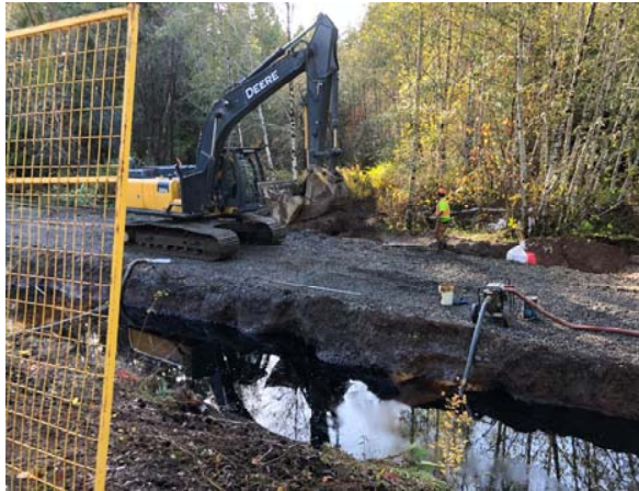
Photo 7. Viewing west towards spilled product in excavated area.
