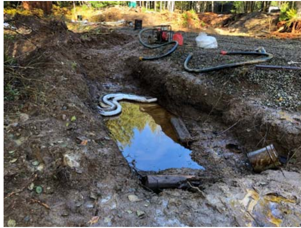
Photo 8. Test Pit location showing spilled product had migrated under the rail tracks towards the wetland.
