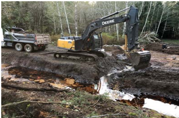
Photo 10. Excavating impacted soil and draining impacted water towards a sump to be transferred into tanks.
