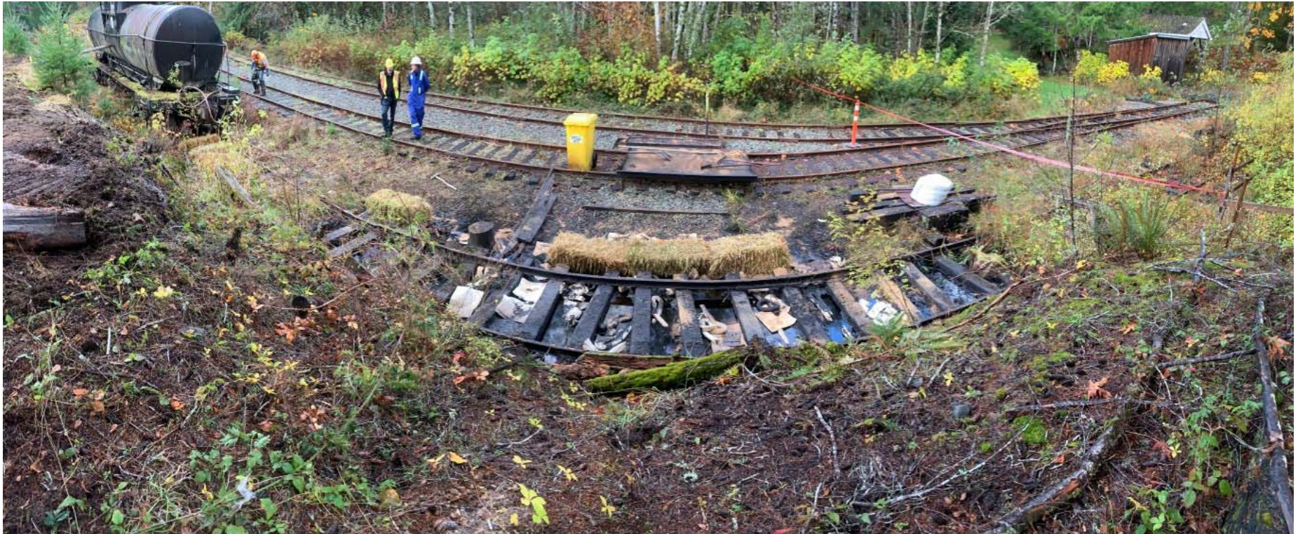
Spill Area After Fuel Rail Tank Moved down Track (October 30, 2020)
