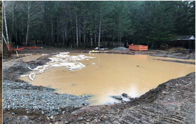
Photo 15. Heavy rains and high groundwater table filled excavation.
