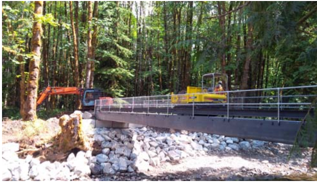
Main trail from Tebo to the second bridge is capped with base material and we will be placing the walking surface materials.
